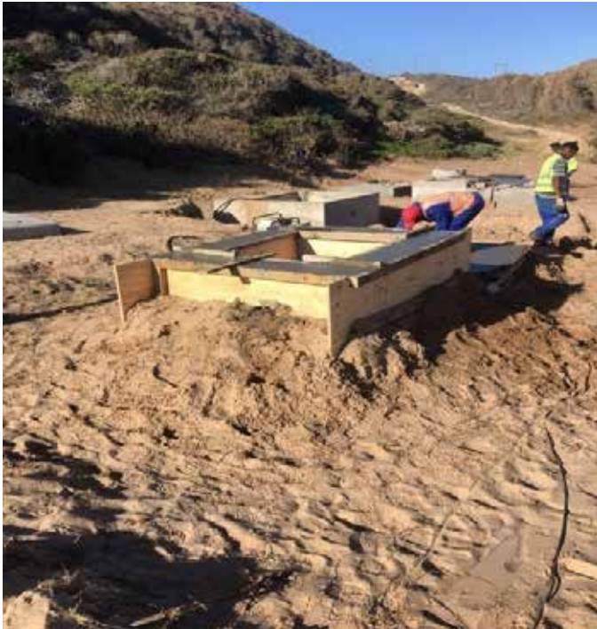
FIGURE 8: Raising a chamber submerged by a sand dune
