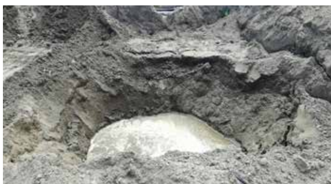
FIGURE 6: High Water Table at the FWF WWTW Tie-in (also existing 900 mm RE pipe to be crossed)
