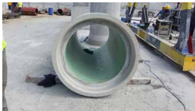
FIGURE 3: RC Pipe with AKS Lining
