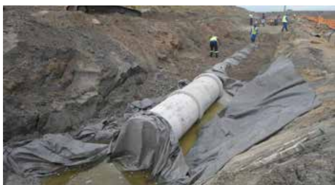
FIGURE 8: Trench Filling up as a Result of Tidal Flow from Swartkops River
