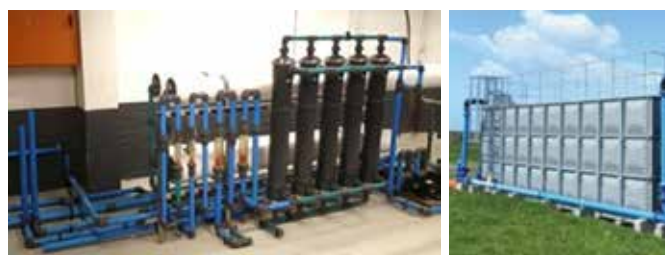
FIGURE 1 (c): Water treatment plant
