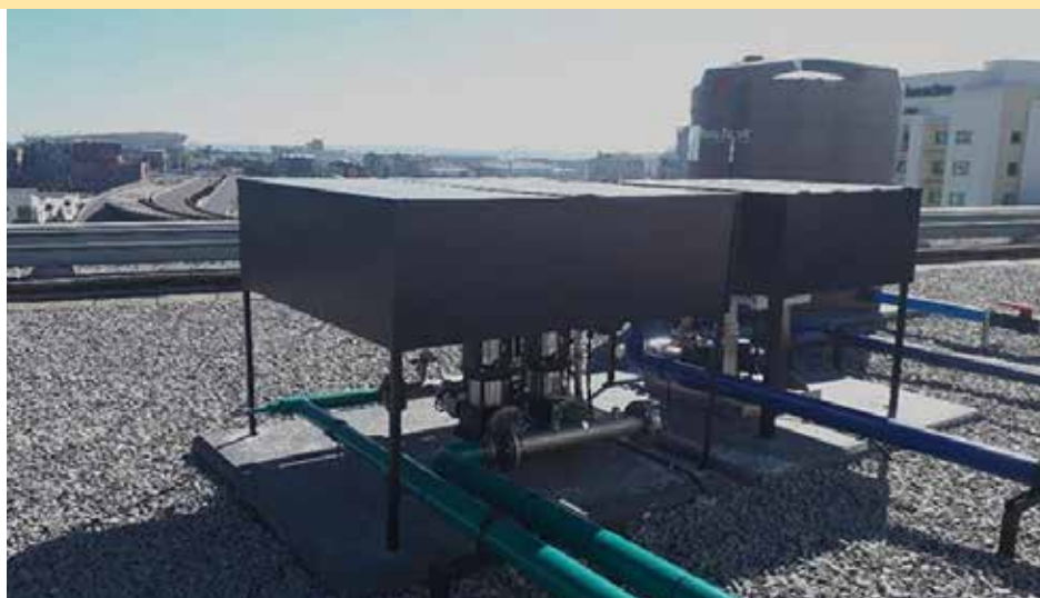
FIGURE 1 (b): Potable and non-potable infrastructure installed at roof level
